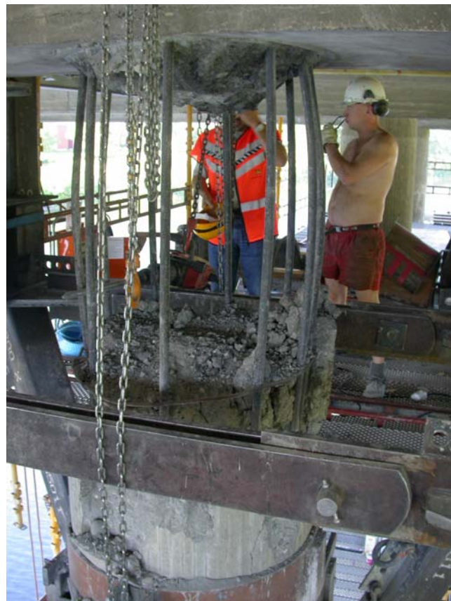
Figure 19: upper part of column 3 in axe 7 where the concrete has been removed.
