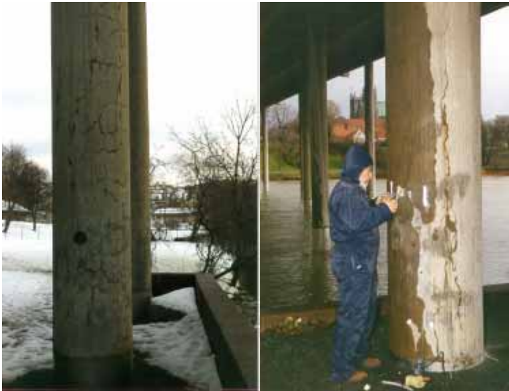
Fig.4: Map cracking and vertical cracks in columns of Elgeseter bridge. Note that the column (right photo) is wet of rainwater on western face (near the man) and dry on eastern face.
