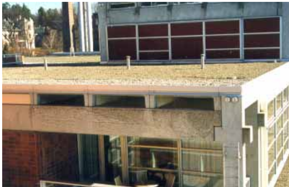
Fig. 10 The Norwegian Veritas House with prefabricated beams and columns. Note the cracked beams in the front
